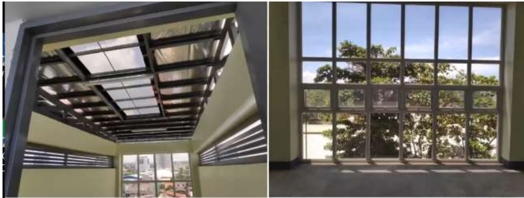
COMPLETION OF IT BUILDING (CONSTRUCTION OF 5-STOREY IT BUILDING PHASE VI) EXISTING CONDITION
