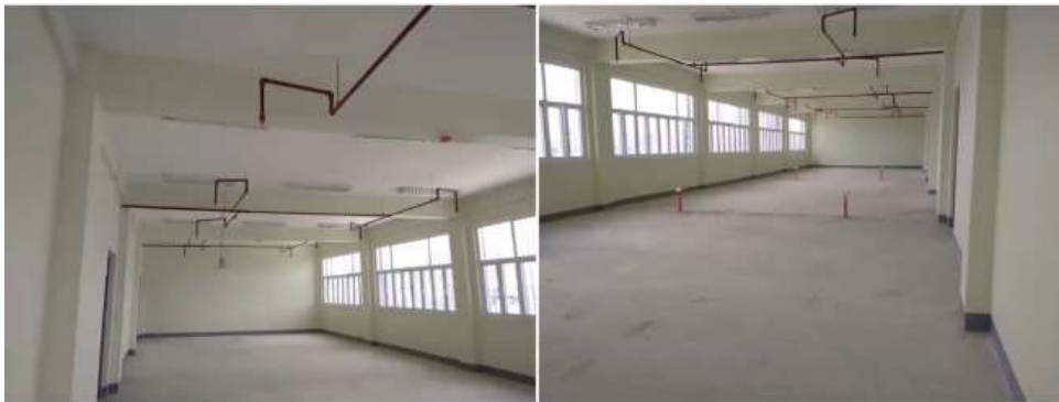
COMPLETION OF IT BUILDING (CONSTRUCTION OF 5-STOREY IT BUILDING PHASE VI) EXISTING CONDITION
